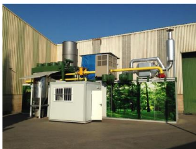
Figure 13: Biomass cogeneration plant in Huedin city (Source: ARBIO – Bioenergy4Business Project)
