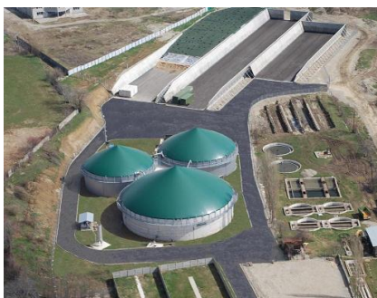
Figure 12: Biogas co-generation plant in Filipestii de Padure (Source: http://www.energyreport.ro )
