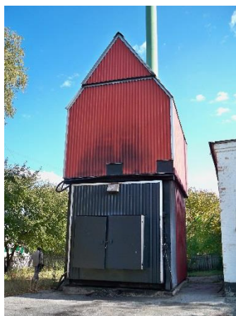
Figure 6 – Straw batch firing boiler in Drozdy
