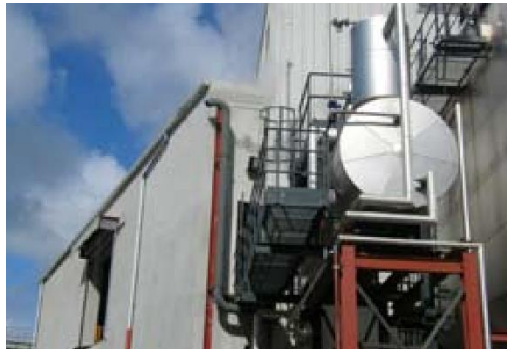
Figure 25: Wood-fueled boiler at Munster Joinery (Source: http://www.seai.ie/Renewables/Bioenergy/Munster_Joinery_Case_Study.pdf )
