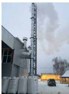
Figure 4 – Woodchip boiler in Kniazhychi
