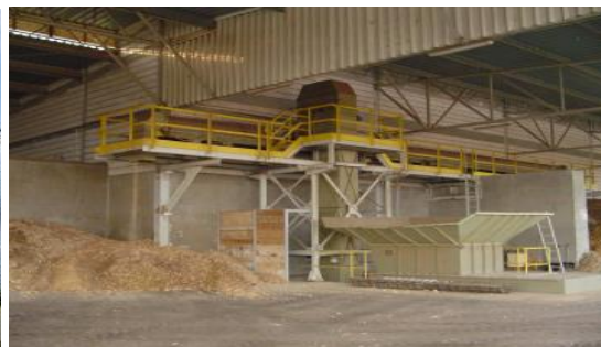
Figure 9: Wood chips storage
